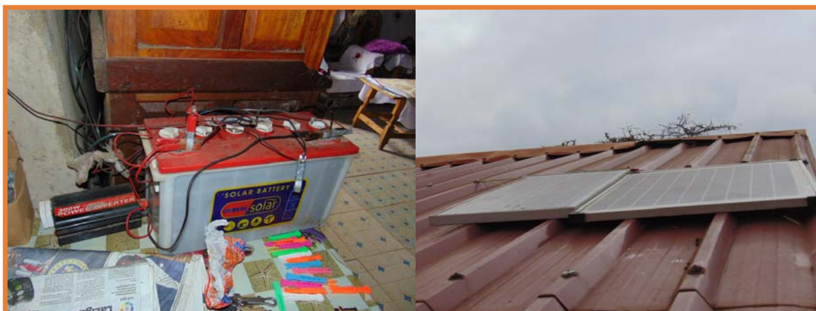
120-Watt-Photovoltaiksystem in Machakos, Kenia; Fotos: Dr. Festus Boamah
